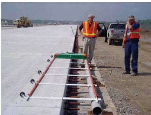
Workers prepare to use MIT Scan-2 to evaluate the dowel alignment in a new pavement joint.
