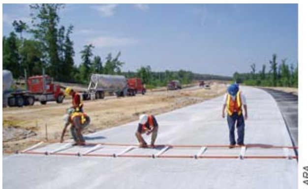
Three workers are using MIT Scan-2 on a U.S. 64 bypass construction project in Knightdale, NC.
